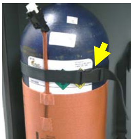
Figure 3a- Tank restraint strap
